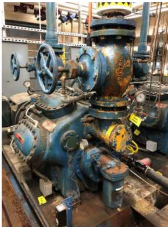
Braemar Ice Plant Equipment
